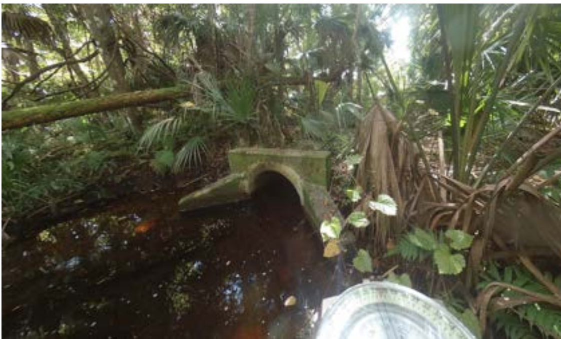
Photo ID# 062421000114MW – 36” RCP from Longmeadow Circle (Echo, 2021)
