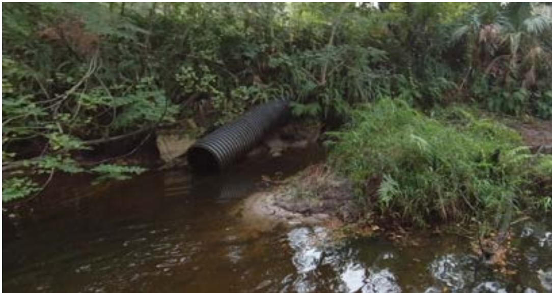
Photo ID# 062421000018MW – 18” CPP from Grove Ct on south bank of River (Echo, 2021)
