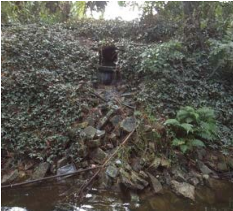
Photo ID# 062421000016MW – 24” CCP from Yew Ct on south bank of River (Echo, 2021)
